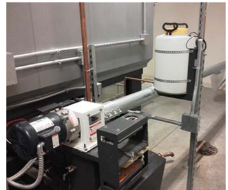
An auger injects pellets into the boiler
