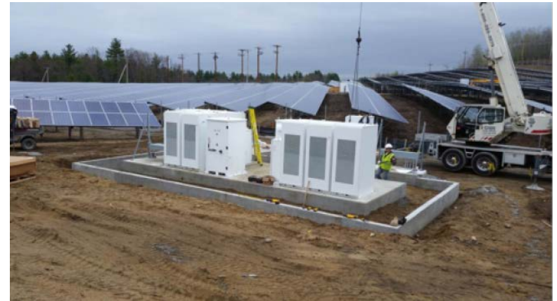
Credit: https://www.3blmedia.com - Tesla Lithium-Ion battery storage system being installed at the National Grid solar site in Shirley, Mass.
