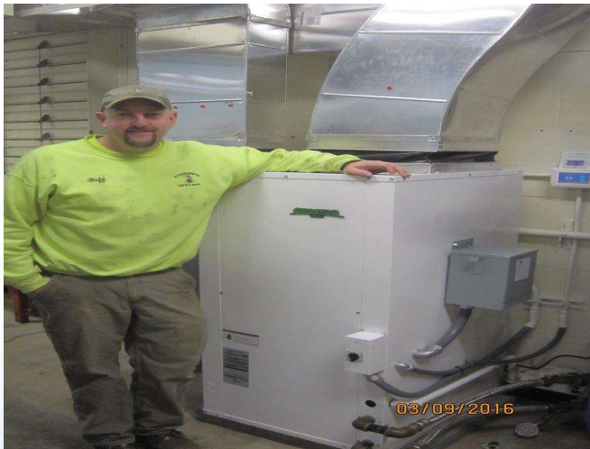
Michael P. Buffoni, Stockbridge Water Superintendent shows off their new heat pump # 2
