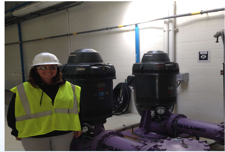
Heather Blakeley, Acting Southbridge Director of Public Works shows off their new effluent pump motors at their wastewater plant
