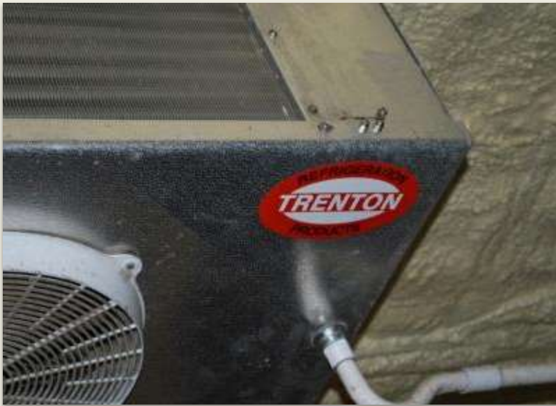
Refrigeration in Each Bay
