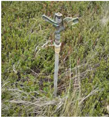
Fig. 1. Impact sprinkler head on metal riser. Photo courtesy H. Sandler.
