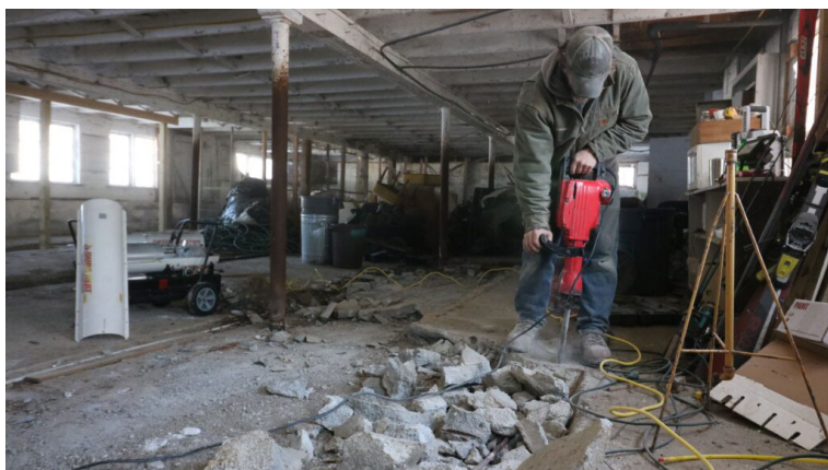
The barn renovation at New Leaf Organics required removing old concrete work which was contracted out. Photo: UVM Ag Engineering
