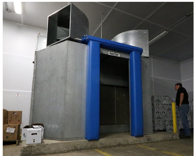
A commercial forced air cooler in a produce distribution facility
