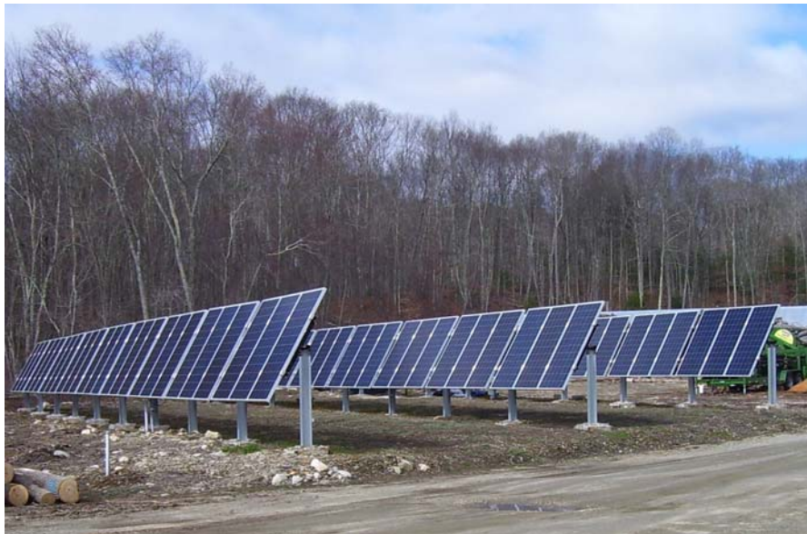
Photovoltaic panels can generate 200 to 300 kilowatts of electricity per year.
