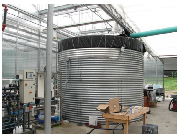
Rainwater Holding Tank
